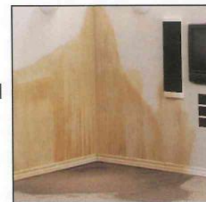
Dampproofing can allow water damage to occur as shown. TUFF-N-DRI assures a dry basement.
